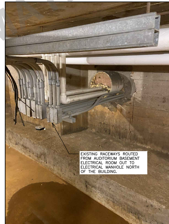
AUDITORIUM BASEMENT ELECTRICAL ROOM (6-5) NO SCALE
